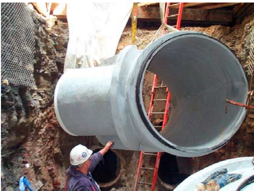
Elsinore Water Main
